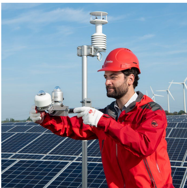
Figure 2 Two SR300-D1 pyranometers, one tilted for Plane of Array (POA) measurement, and another mounted horizontally for Global Horizontal Irradiance (GHI) measurement.
