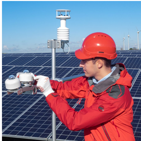
Figure 0.3 Two SR30 spectrally flat class A pyranometers with digital output for GHI (Global Horizontal Irradiance) and POA (Plane of Array) PV monitoring measurement
